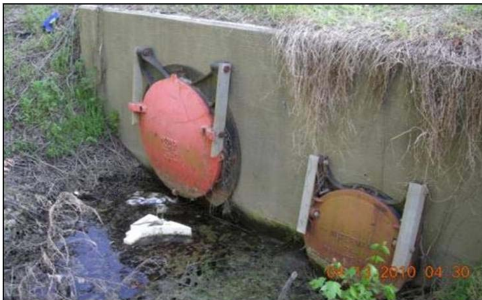
Figure 1.9: Flap Gate Backflow device on culverts
