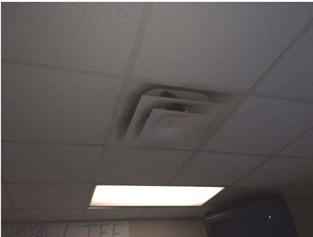
HVAC supply registers appeared to be clean. Register over teacher's desk was blocked with cardboard.
