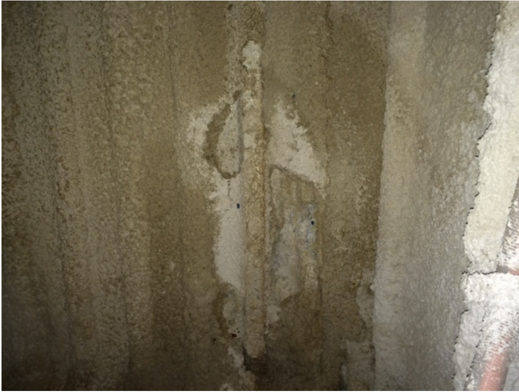
Water damaged fireproofing above suspended ceiling in 3320.
