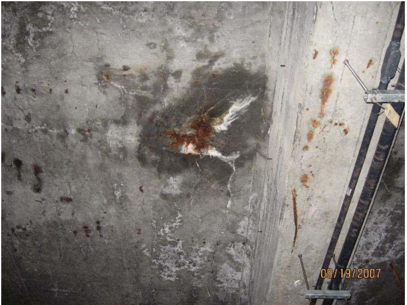
Beginning of a punch-through of the roadway deck
