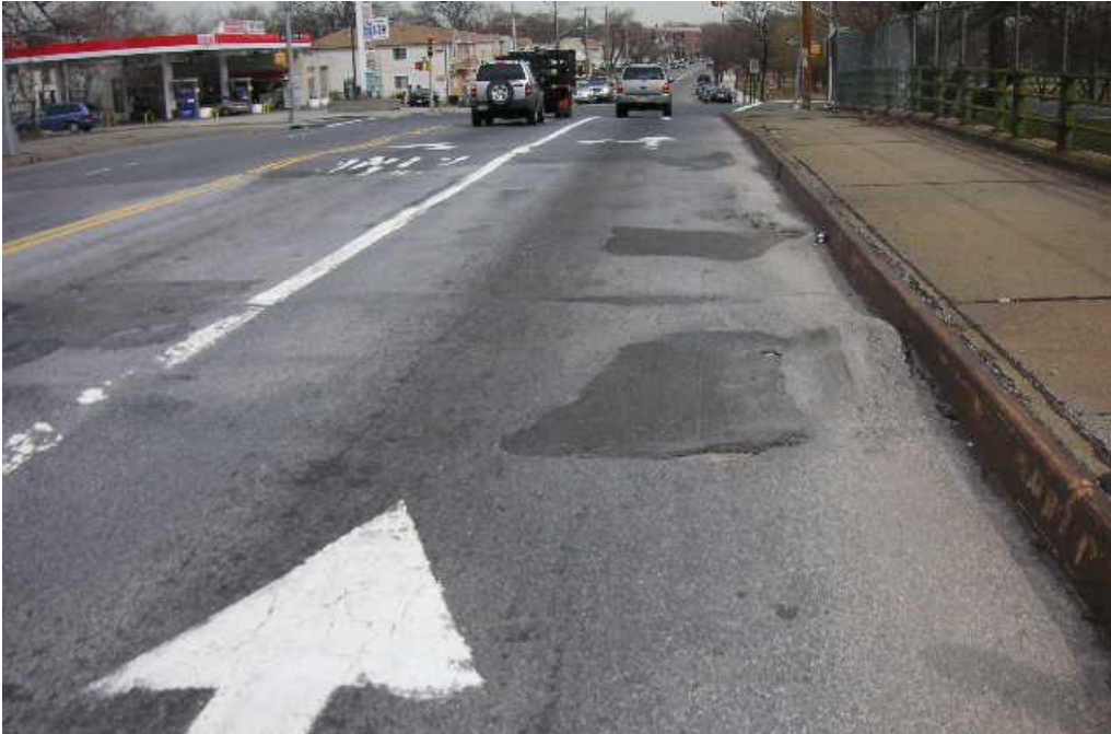
Top of bridge: Deck holes covered by asphalt repairs
