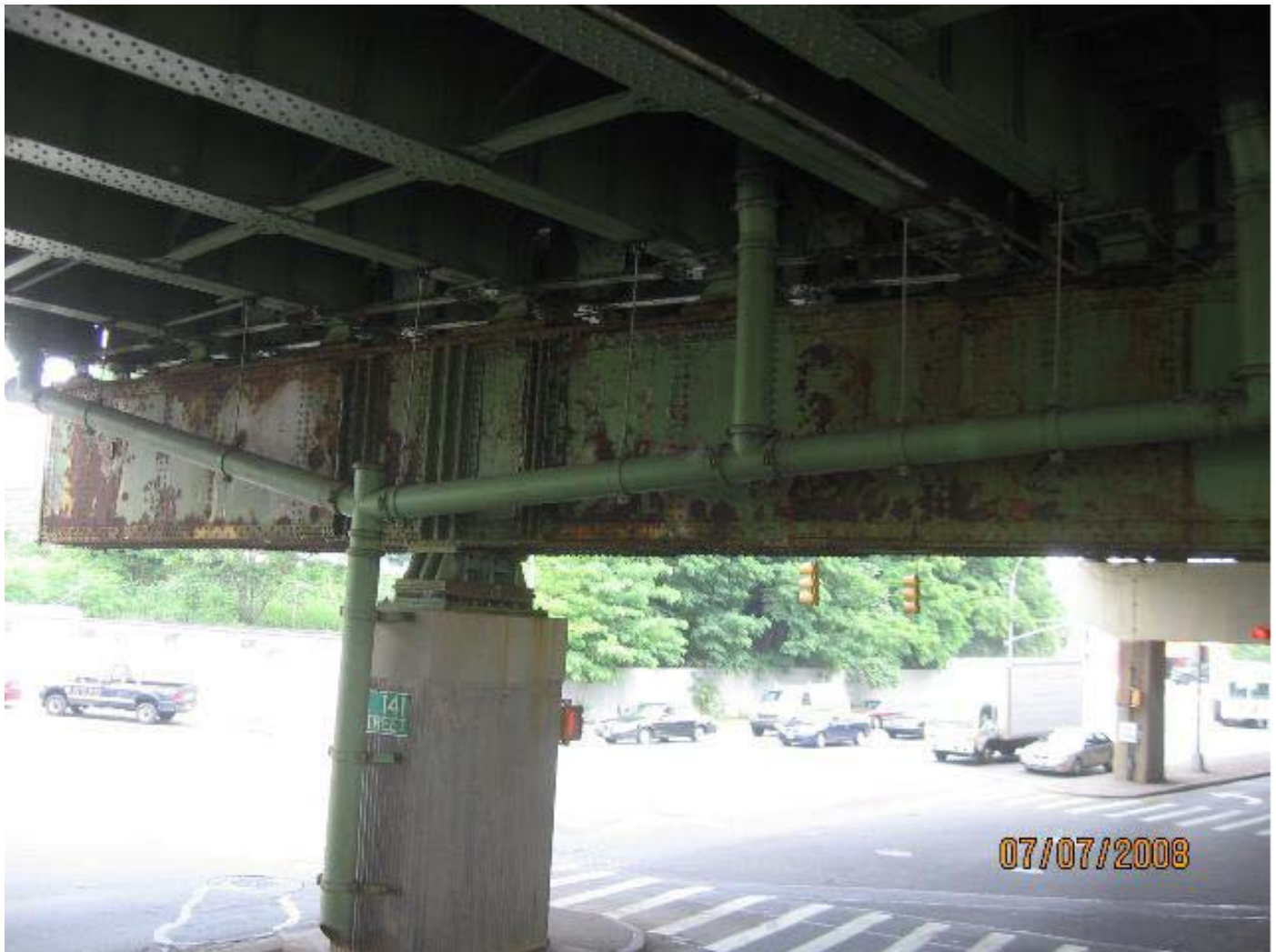
Failed joint causing floor beam deterioration
